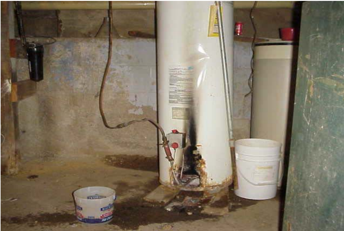
Non operational water heater - gas line not code - burner roll out
