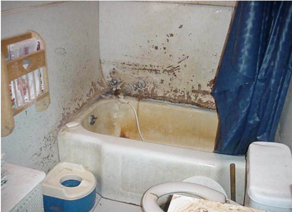
Small bathroom stained & drywall rotted
