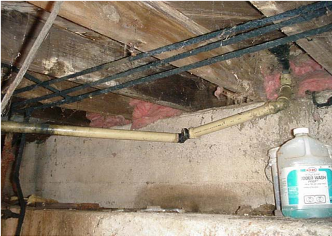
Water lines covered by ½” black mold
