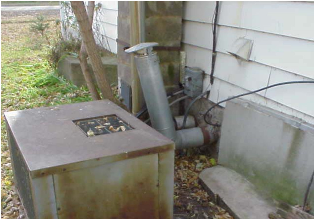
Furnace flue vent dangerous
