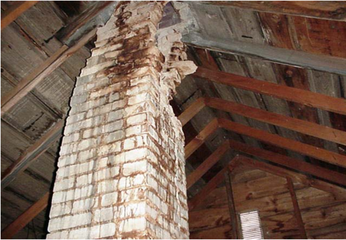
Chimney coming down in attic
